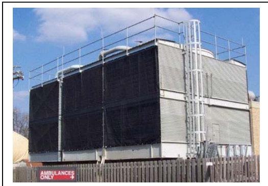
Air Intake Filters Protecting Large Cooling Tower
