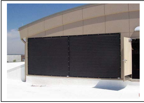
Louver Filters Protecting Internal Filters on Air Handling Unit
